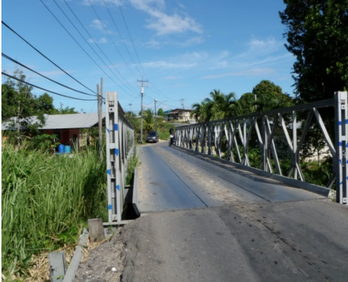
Figure 3. The Bailey bridge before the Construction of the Bridge B1/1 Freeport Todd's Road.
